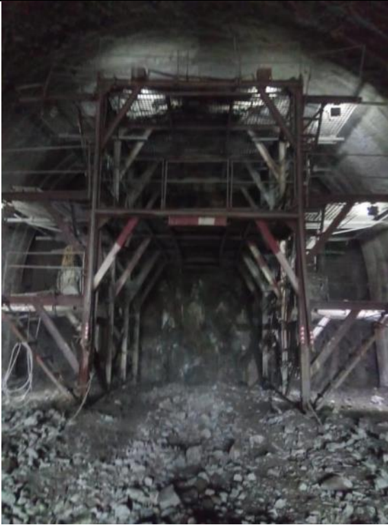
#10 Tunnel/ Accident place
